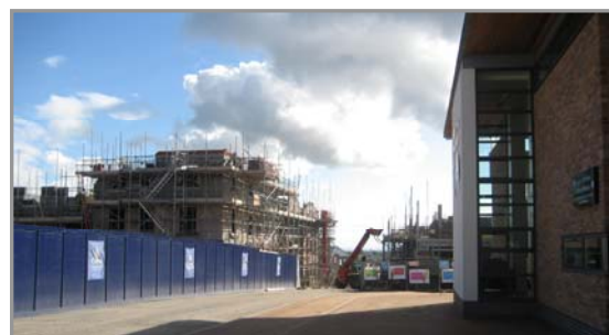
Village centre and care home currently under construction opposite the new primary school and community hub
