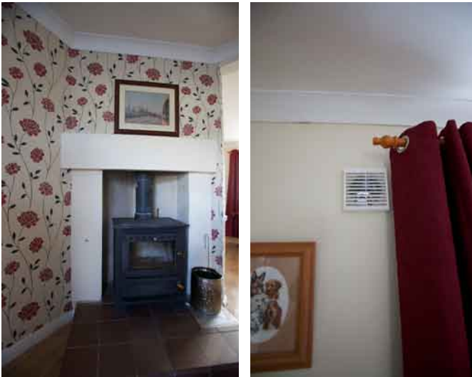
UK regulations require an uncontrolled air supply for a wood burner. The M&E contractor installed an air-brick to deal with this (somewhat compromising air tightness).
