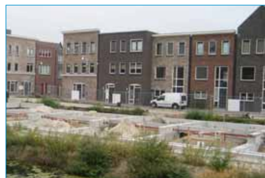
Foundations including ground source heat pumps are provided by the public private partnership before the sites are handed over to developers
